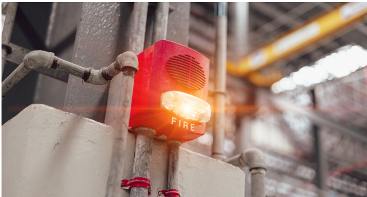
Emergency & Safety Lighting
